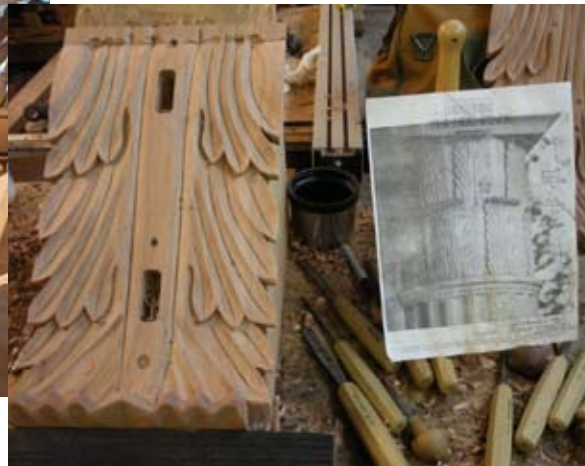
Acanthus-carved redwood panels with a photo of the Hermitage column capitals on right.
